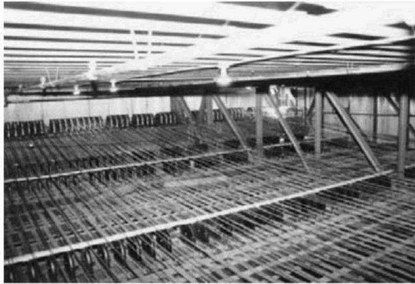
Fig. 3.24. Sag bars on top of grid-mounted loft blocks
