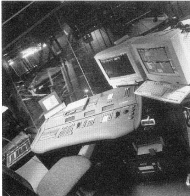
Strand 500 desk installed by Northern Light at the Lowry Theatre in Salford
