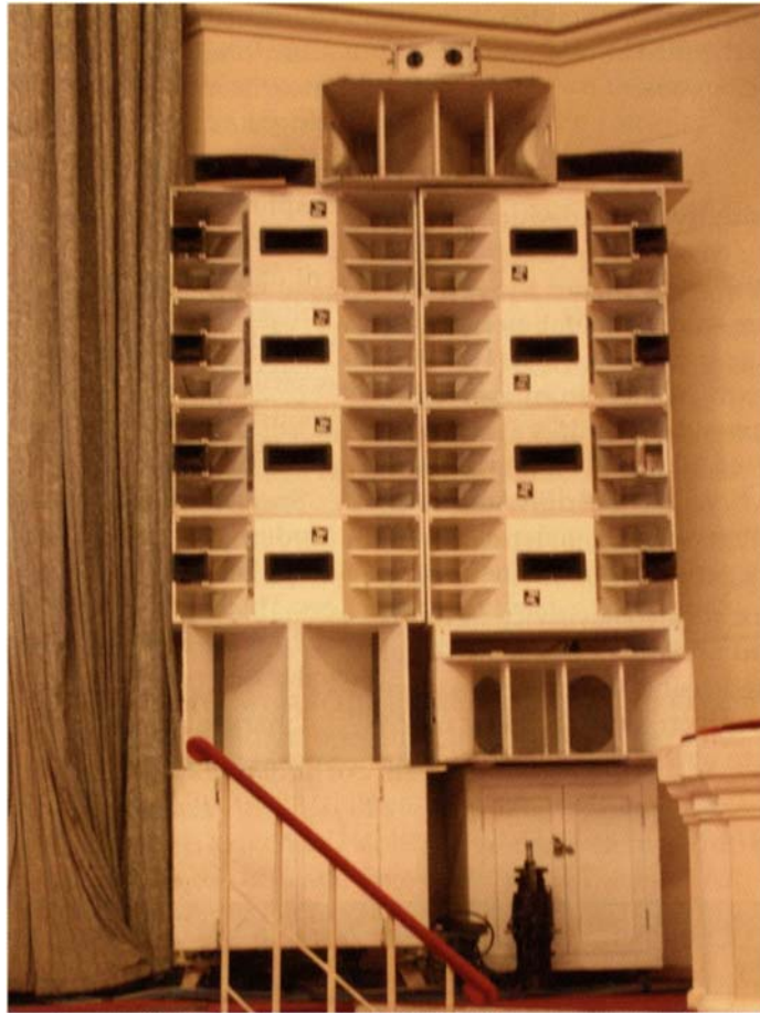
This loudspeaker escaped from its garage. This is not considered an engineered system (photo courtesy of Dave Lawler)
