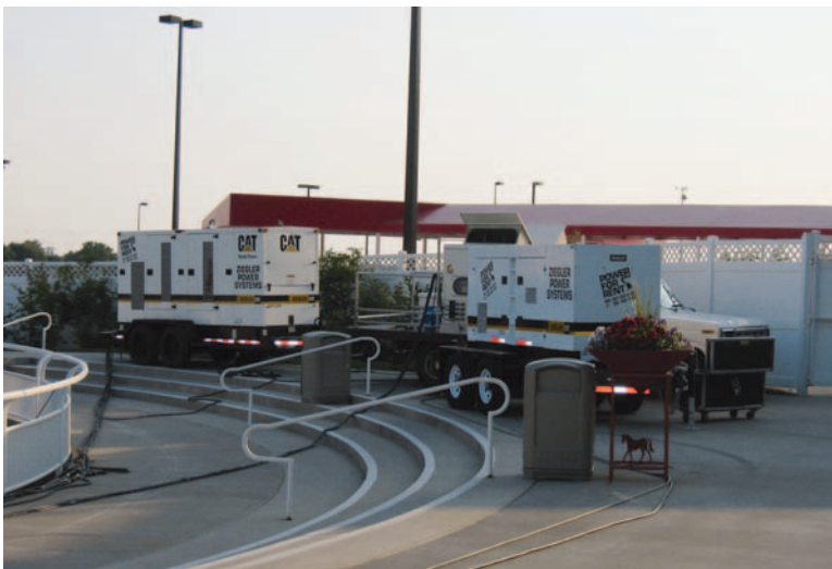
FIGURE 12.12 Portable generators. (Photograph by Paul Dexter.)
