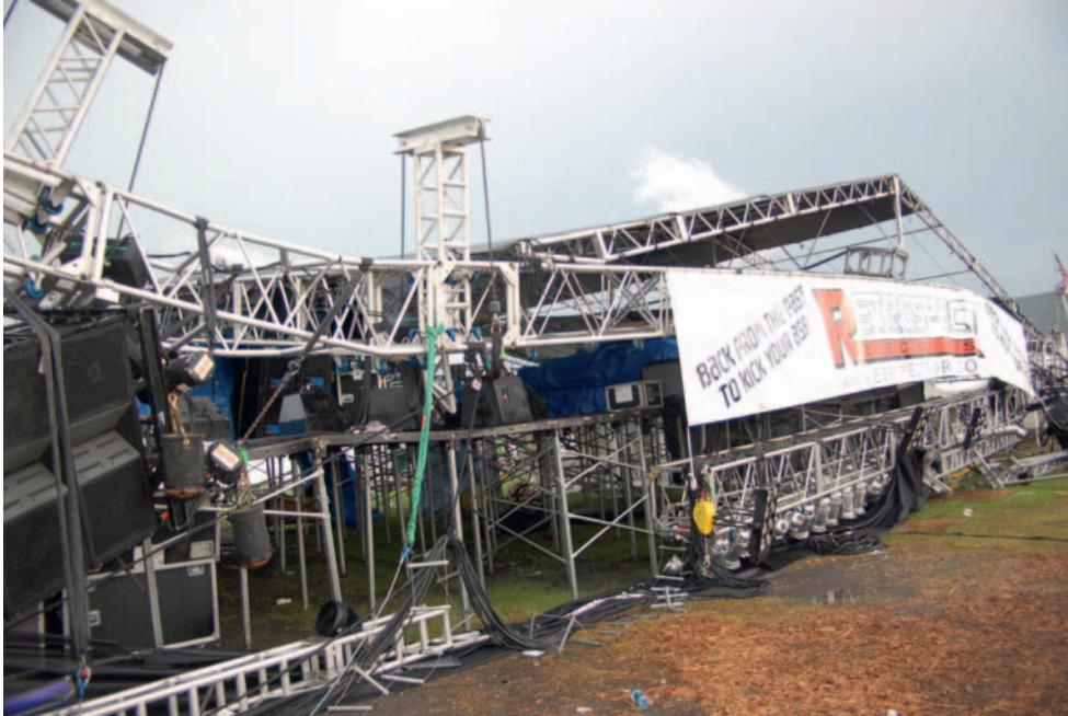
FIGURE 9.8 Truss collapse at Rocklahoma caused by storm in Summer 2008. (Photograph by Robin Alvis.)
