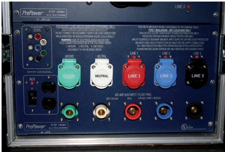
Figure 6-18 120/208 VAC four-wire plus ground electrical distribution panel.
